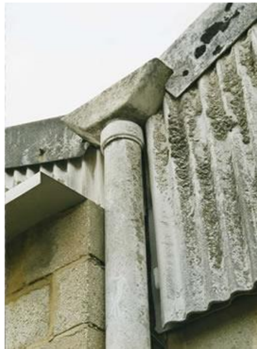
Asbestos cement downpipe, hopper and profile sheet
