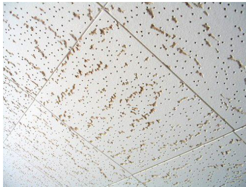
Asbestos containing ceiling tiles
