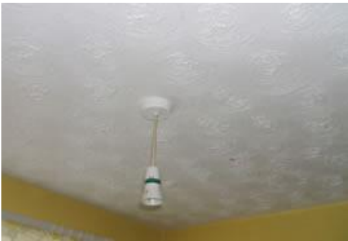
Asbestos textured coating
