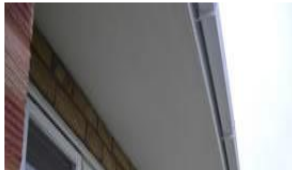
Pieces of Asbestos Insulating Board (AIB)
