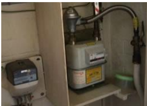
Asbestos panelling around a gas meter
