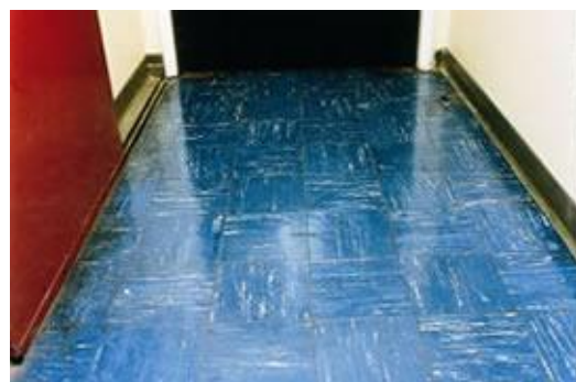
Asbestos containing floor tiles in a corridor
